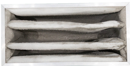
The filter that needs to be replaced
